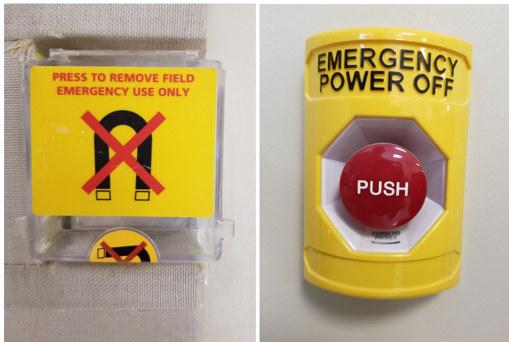
Figure 2b. Emergency Response Buttons inside the 7T Magnet/Scanner Room
