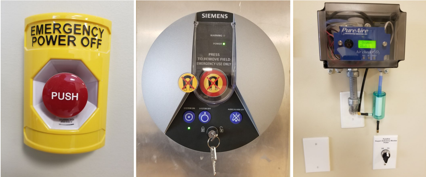
Figure 1b. Emergency Response Buttons inside the 7I Console/Control Room
