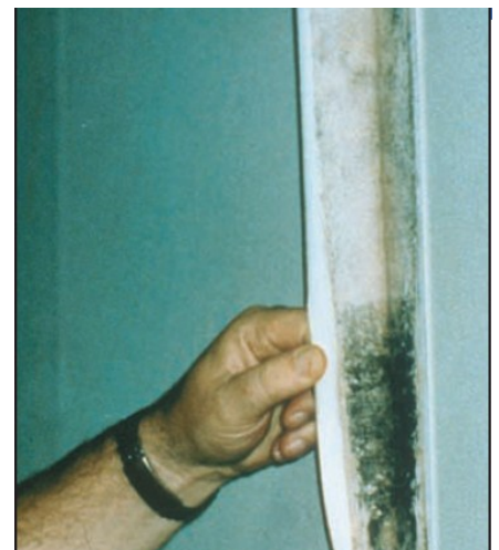
Mold growing on the back side of wallpaper.
