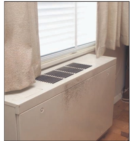
Mold growing on the surface of a unit ventilator.
